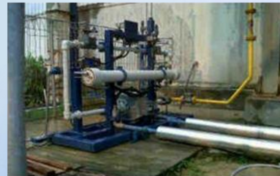
Peralatan Penerima CNG Pressure Reducer Station (PRS) and Gas Metering System
