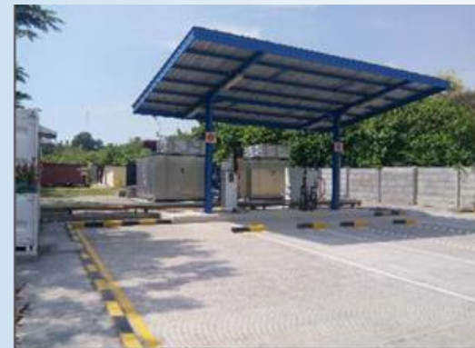
CNG Compressors and Filling Stations
