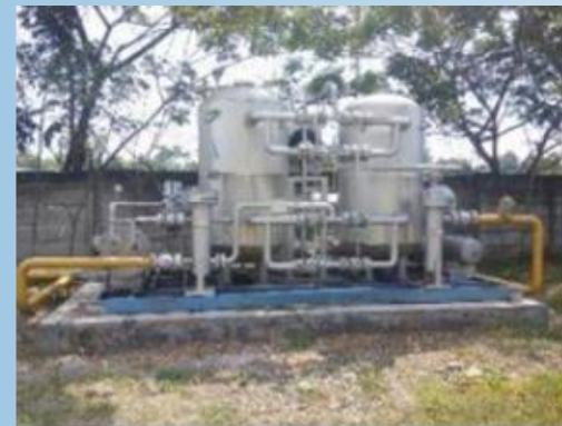
Gas Dryer Unit
