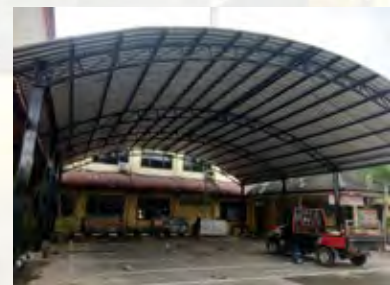
CSR Plat Rembang : Bantuan pembuatan atap kanopi parkir polres Rembang 21-6-21 Rembang Plant CSR Construction of canopy to parking area of Rembang Office Station
