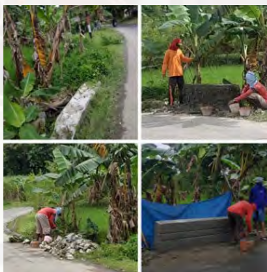
CSR PLAT REMBANG : Bantalan gorong- gorong Dk. Kedung Sapen Ds. Jatihadi, Kec. Sumber Rembang 2-2-21 Water channel construction at Dk Kedung Sapen, Jatihadi Village, Sumber Sub- District, Rembang
