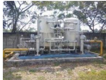
Gas Dryer Unit
